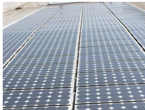
Figure 6: Modules after cleaning
